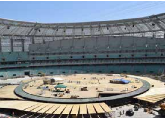
Red Circle Mechanical Equipment Frame Works
